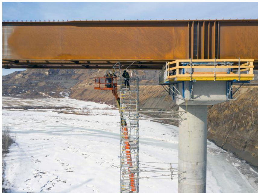
Figure A-10 Girder installation is complete, and workers remove scaffolding from the Halfway River bridge (March 2021)
