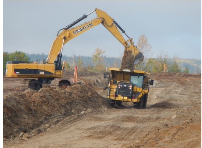
Excavation of material; part of the north bank at the Site C dam site
