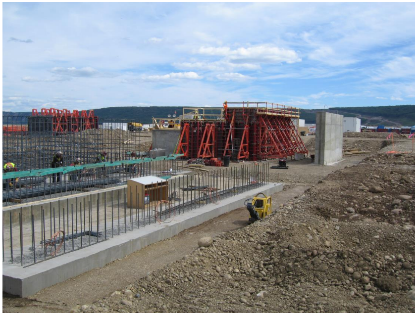
Figure A-4 North Foundation for Roller-Compacted Concrete Batch Plant. Photo taken July 29, 2016
