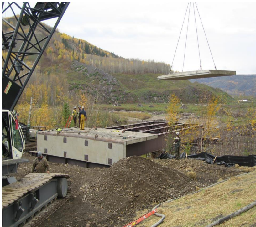
Figure A-12 Installing Bridge Deck Panels on the Moberly River Construction Bridge
