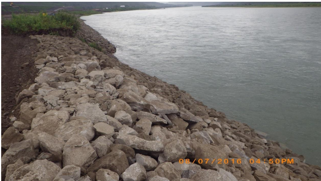
Figure A-8 Right River Bank – Erosion Protection On-going Works between Right Bank Cofferdam Sta. 0+900 and Sta. 1+000 (4Evergreen). Photo taken August 7, 2016
