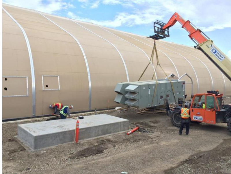
Figure A-3 Crew Installing Air Handling Unit for the Gymnasium. Photo taken July 25, 2016
