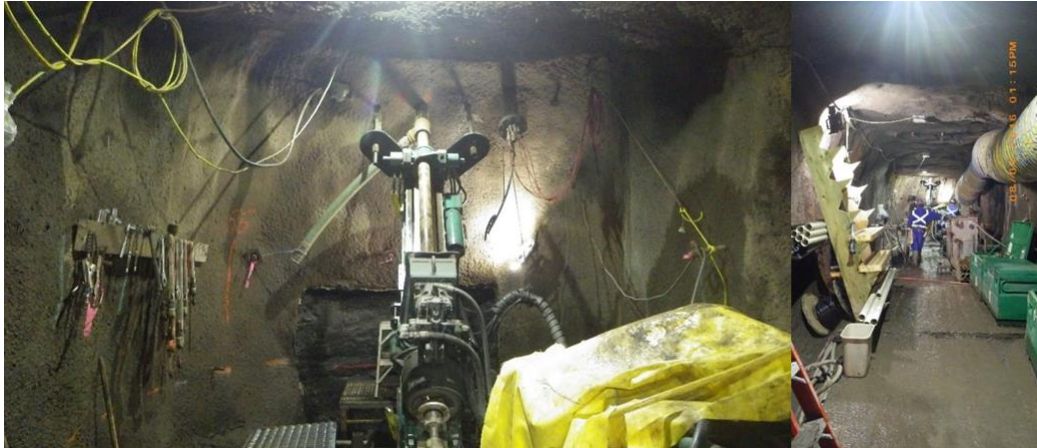
Figure A-6 Right Bank Adit No. 5 – In progress Drilling for Instrumentation. Photo taken August 4, 2016
