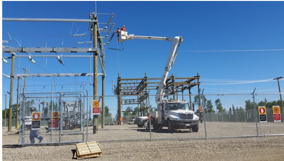
Figure A-1 Installing 138 kV Drops into Site C Temporary Substation. Photo taken July 2016
