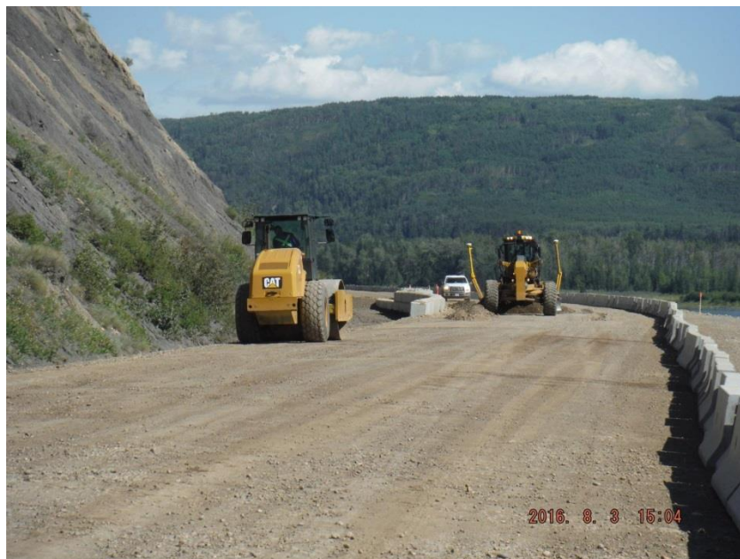
Figure A-5 Looking Easterly on River Road. Working on Road Maintenance. Photo taken August 3, 2016
