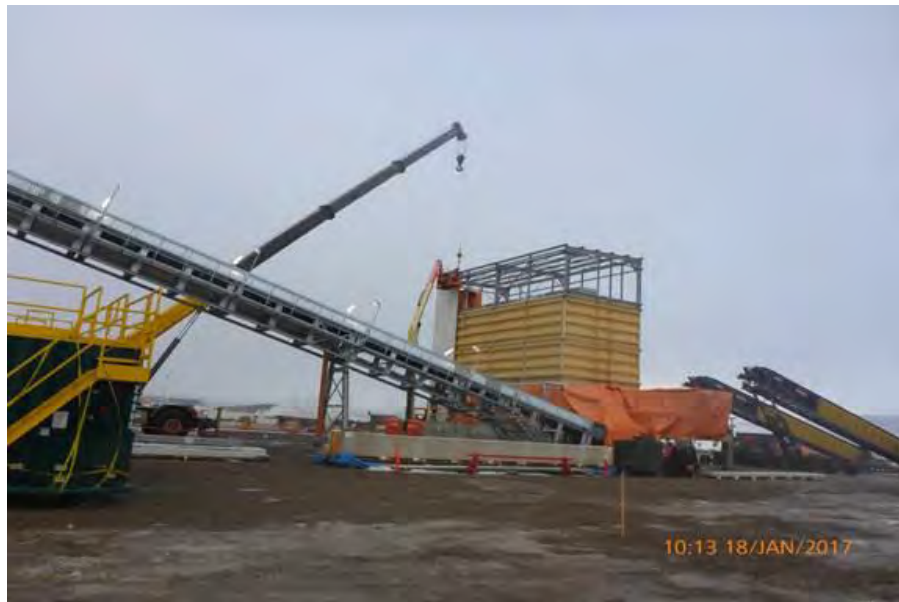
Figure A-2 Area 21 - Installing Cladding at Conventionally-vibrated Concrete Plant #6. Photo taken January 18, 2017.
