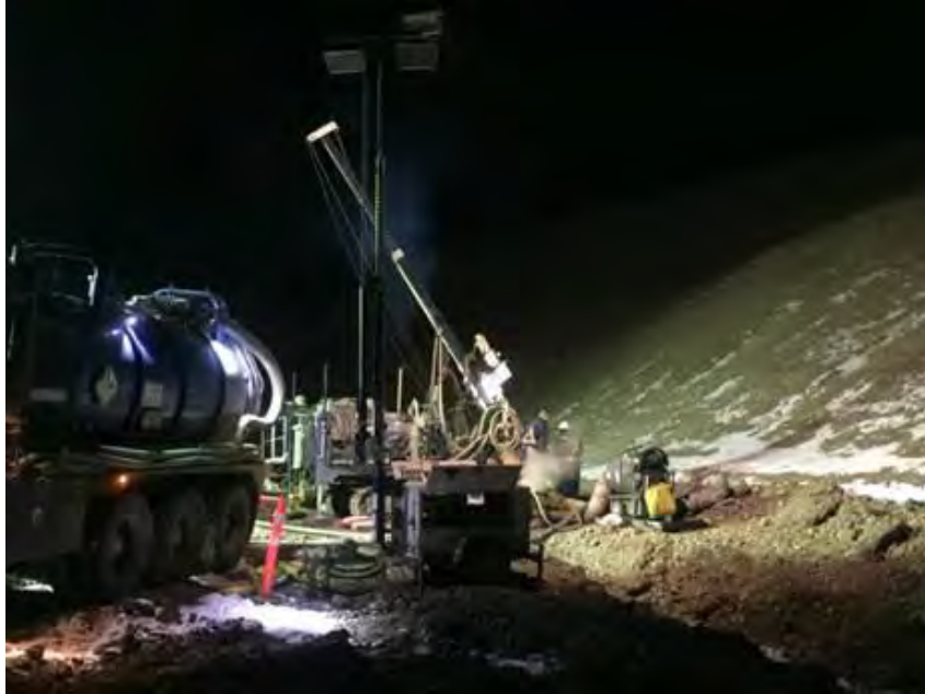
Figure A-7 Foundex on Site Drilling for Instrumentation at the North Bank Slope Failure Area. Photo taken March 1, 2017.
