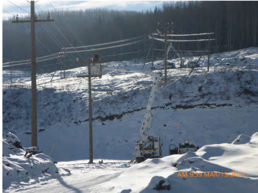
Figure A-9 Transmission Line Right of Way Stringing Conductor Line. Photo taken March 13, 2017.
