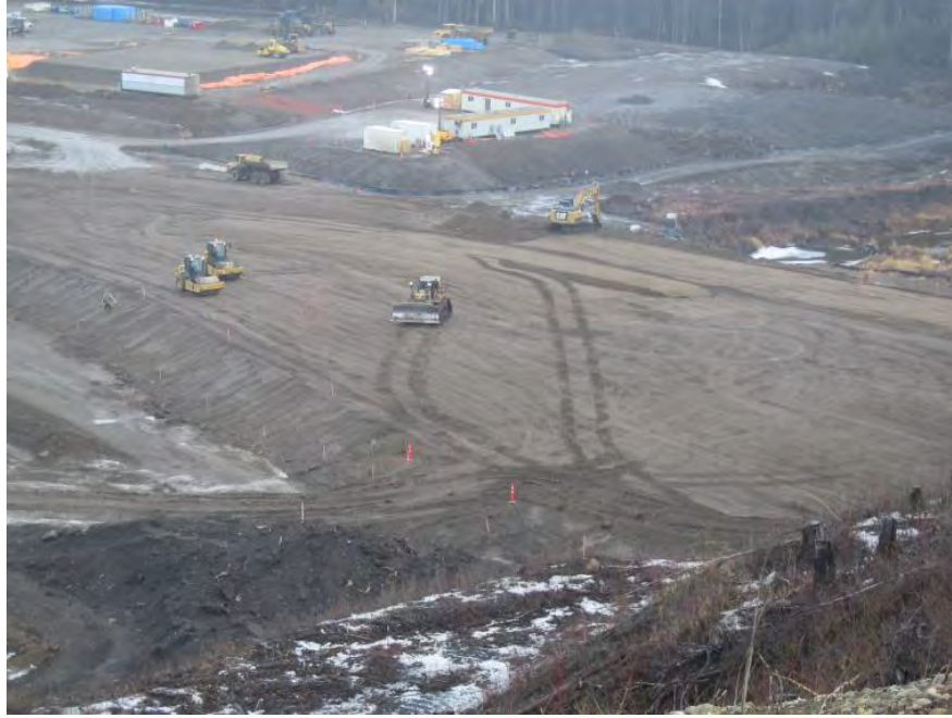
Figure A-5 South Bank Initial Access Road - Facing Northeast. Photo taken February 17, 2017.
