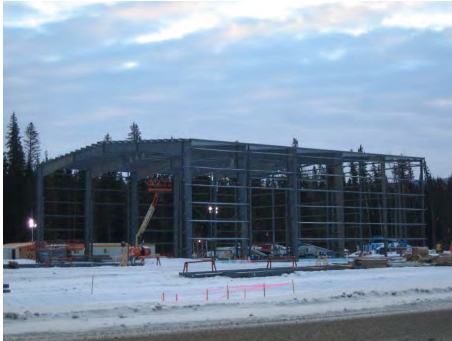
Figure A-1 River Island Laydown Truck Maintenance Shop; Working on Structural Steel. Photo taken January 4, 2017.
