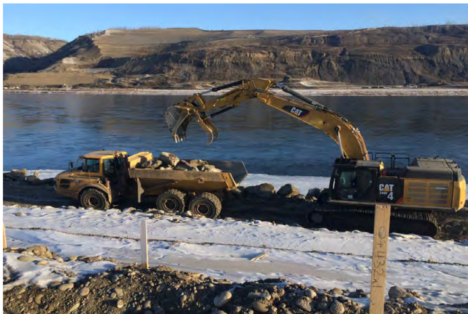
Figure A-4 Right Bank Cofferdam – Facing North; Excavator Loading Rock Truck with Excess Rip Rap. Photo taken February 12, 2017.
