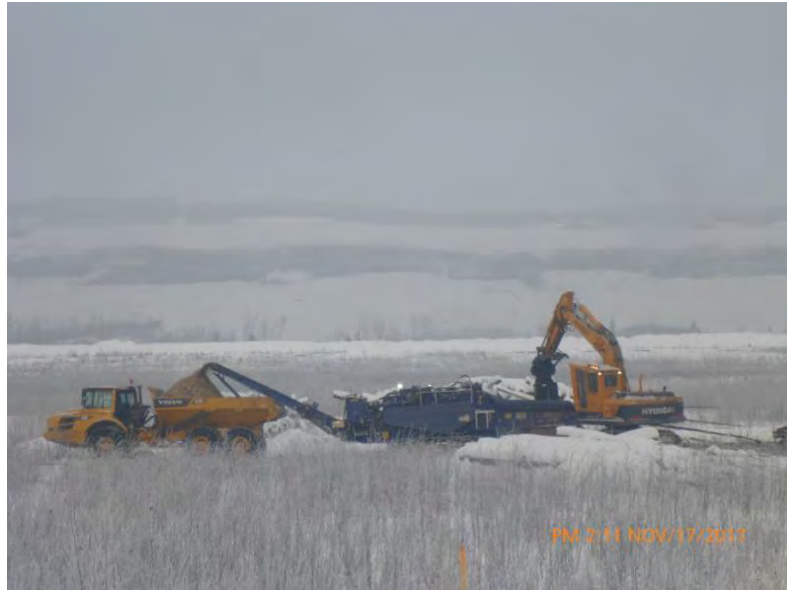
Figure A-5 Generating Station and Spillway Area southwest Section - Mulching of Woody Debris Continues. Photo taken November 17, 2017.
