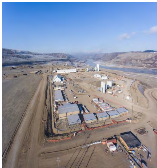
Figure A-4 Batch Plant Area on the South Bank. Photo taken November 3, 2017.
