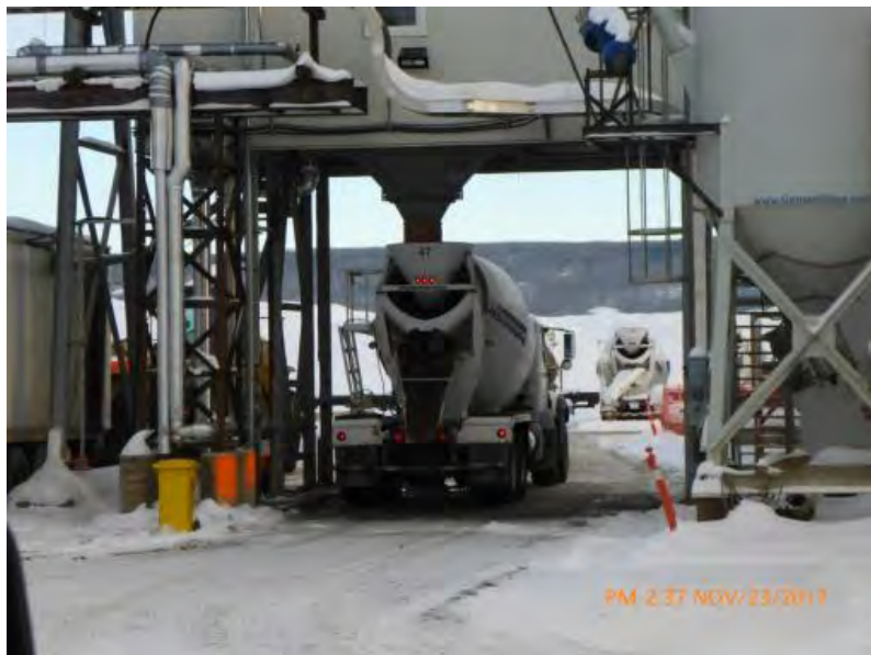
Figure A-6 Plant Producing Shotcrete for the Right Bank Drainage Tunnel. Photo taken November 23, 2017.
