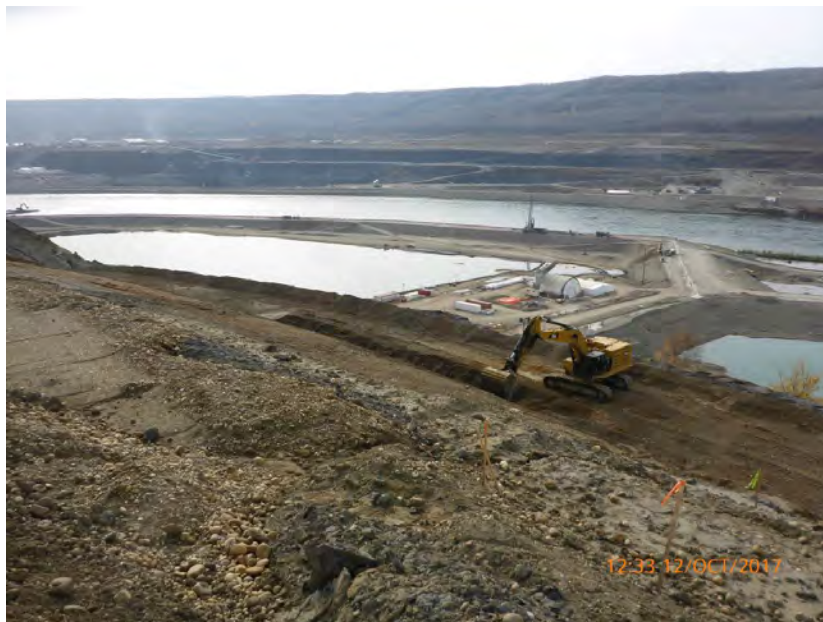
Figure A-2 Left Bank Excavation - Excavator Cutting Ditch along Bench 0-2 Slope. Photo taken October 12, 2017.
