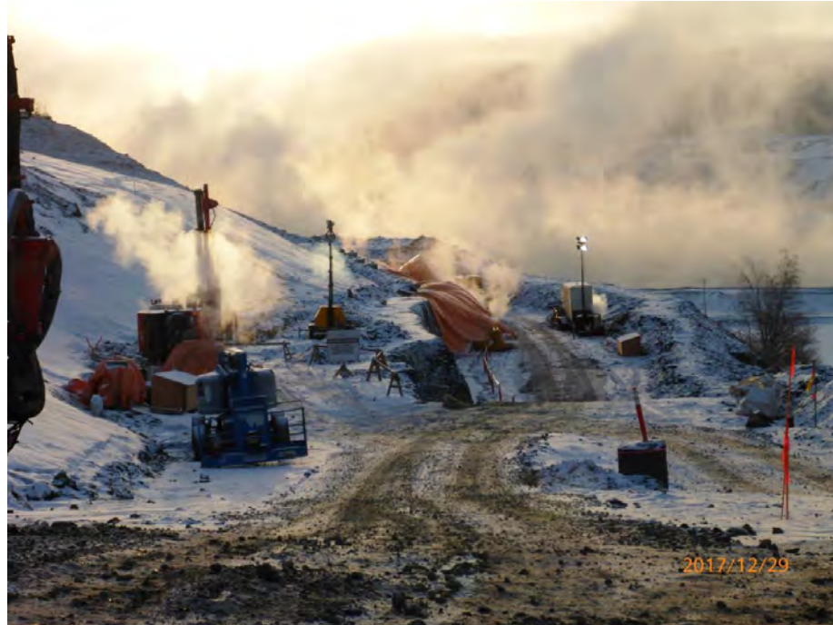
Figure A-9 Inlet Portal – Continued to Heat and Hoard the Shotcrete Face on Bench O. Photo taken December 29, 2017.
