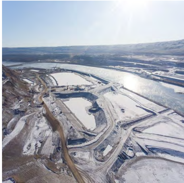
Figure A-3 Aerial View of the North Bank, with Cofferdams and Laydown area, Looking Southeast. Photo taken November 3, 2017.
