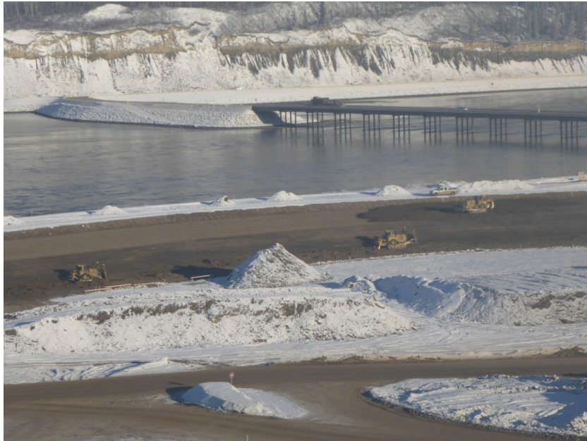
Figure A-7 Relocated Surplus Excavation Materials R6 - Facing Northeast. Photo taken December 2, 2016.
