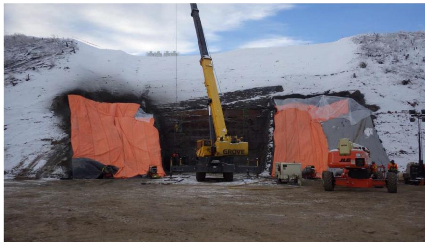
Figure A-6 Right Bank Drainage Tunnel Facing South – Prepared Rock Surface Covered and Heated prior to Shotcrete Application. Photo taken December 2, 2016
