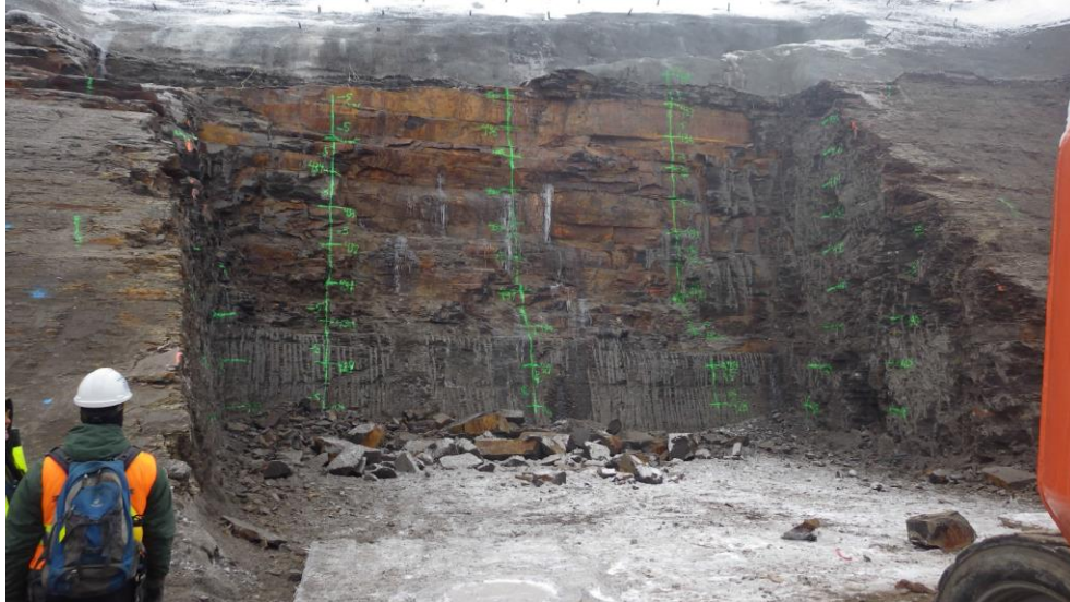
Figure A-3 Right Bank Drainage Tunnel Portal - Face Was Cleaned and Marked for Mapping. Photo taken November 25, 2016
