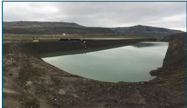
Above: Sediment pond at the Site C dam site. Sediment ponds are a best practice in sediment control. During a rain event, these ponds capture runoff that may contain eroded soil. The pond allows the sediment to drop to the bottom and keeps the water exiting the pond clean.
