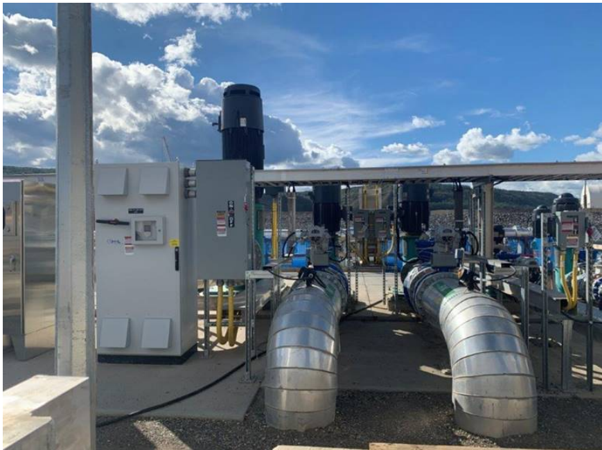
Large pumps on the exterior of the fishway
