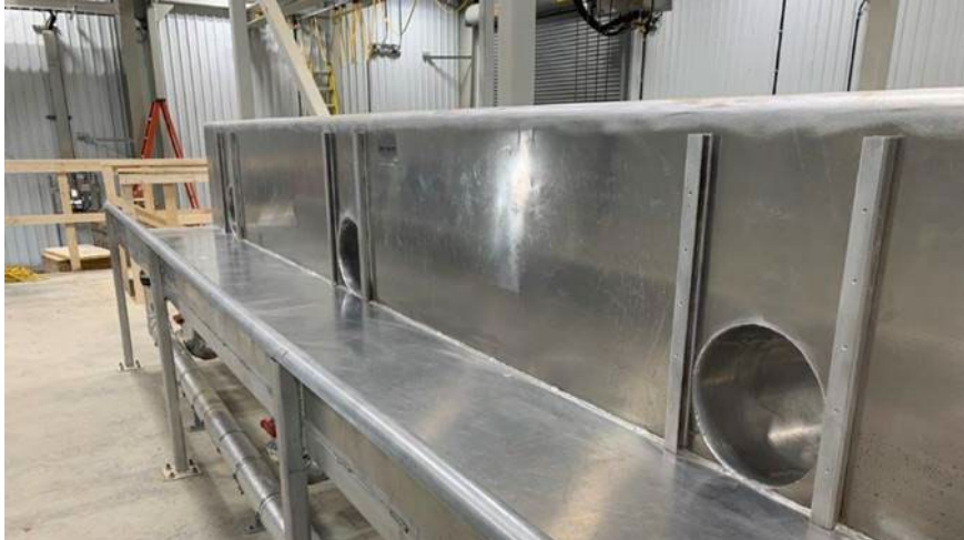
Fish sorting table: This is one of the many components of the fishway that will have flowing water very soon
