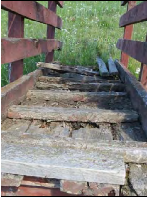
Photo 7. Cattle-handling infrastructure needing repair
