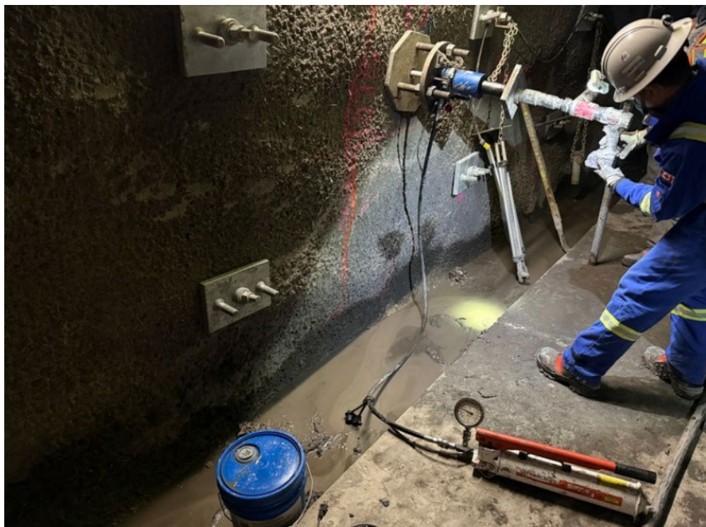
Figure A-17 Right Bank Drainage Tunnel – Rock bolt Torque and Tension Test (December 2025)
