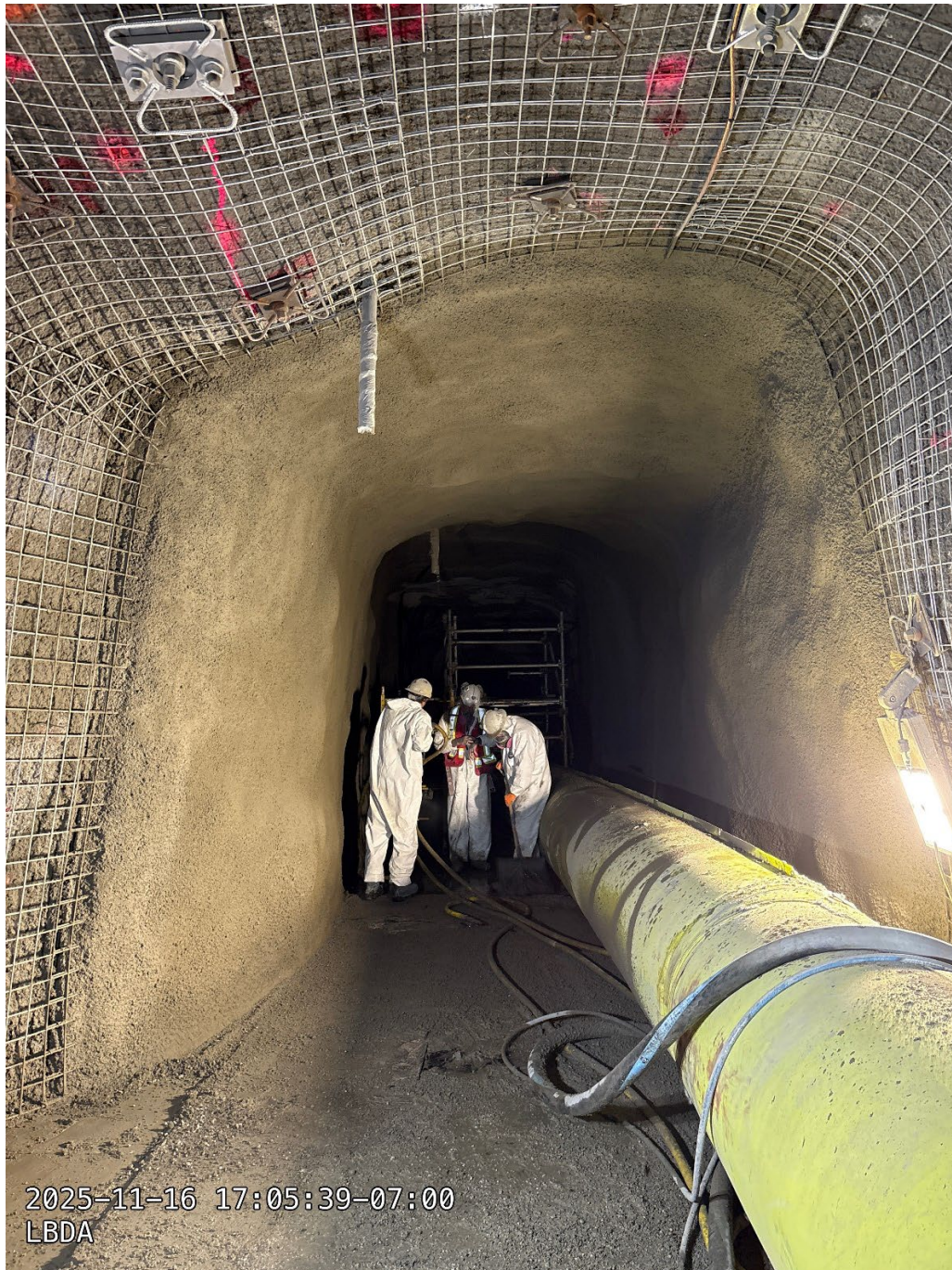
Figure A-9 Left Bank Drainage Adit - Production bolting, mesh and shotcrete placement (November 2025)
