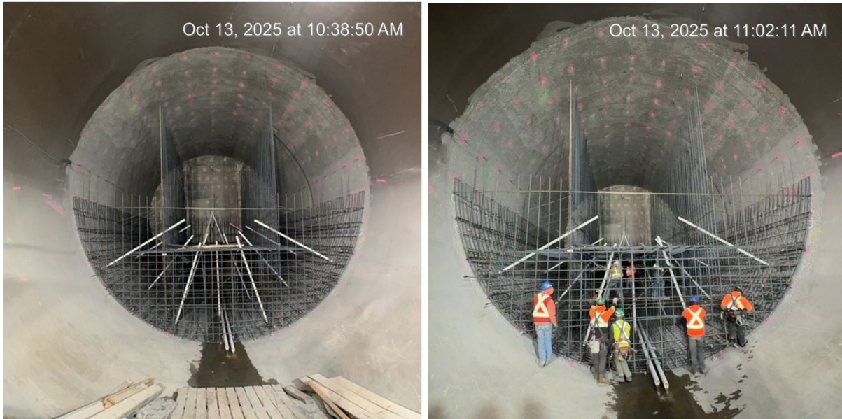
Figure A-7 Construction of the concrete plug for the Diversion Tunnel 1 backfilling. Carpenters are installing formwork coil rods and crews are completing rebar installation. (October 2025)
