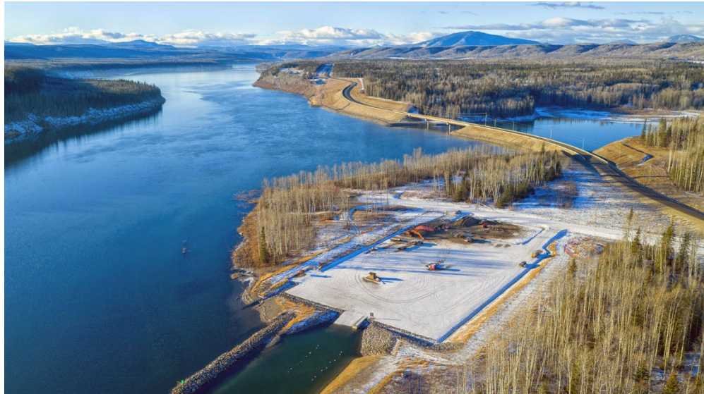
Figure A-16 Construction Activities in Progress at the Lynx Creek Boat Launch (December 2025)
