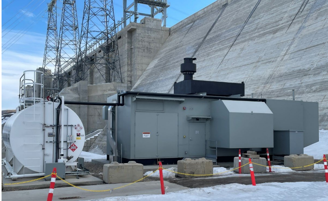
Figure A-24 Powerhouse Diesel Generator (January 2026)
