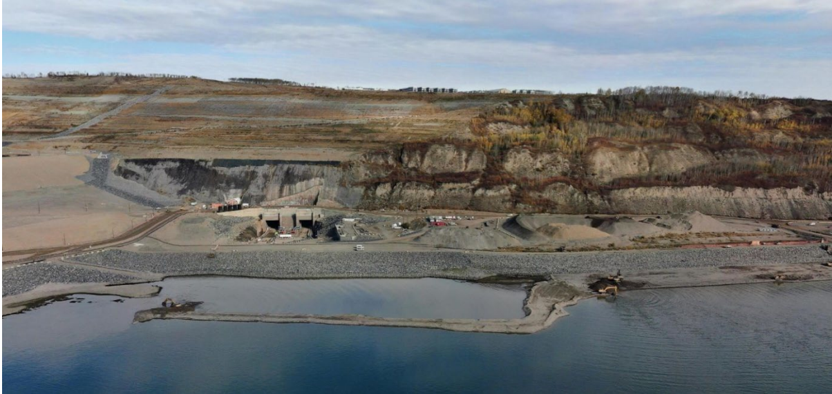
Figure A-5 In-river excavation work. This work will improve fish habitat, reduce fish stranding risk, increase plant discharge capacity and provide gravel for the diversion tunnels. (October 2025)
