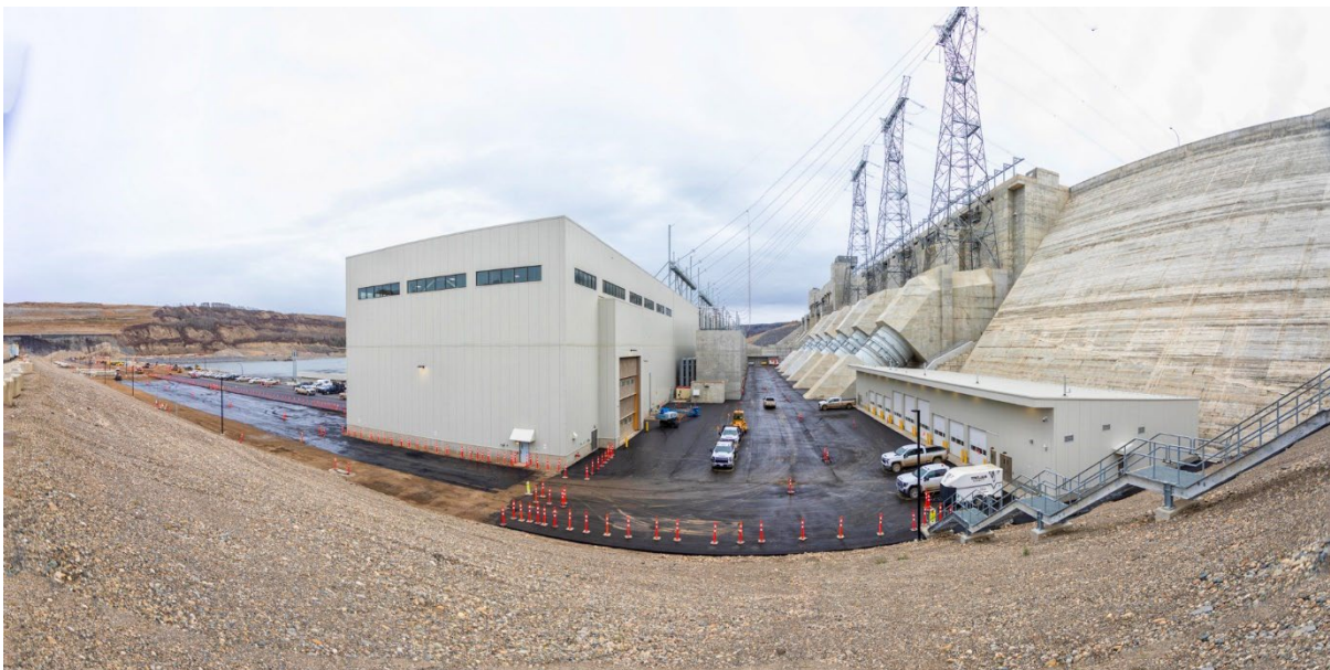
Figure A-4 Transformer Yard (October 2025)
