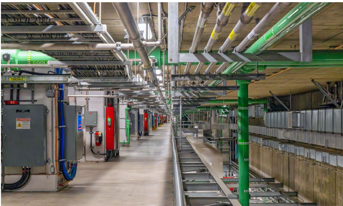
Figure A-23 Turbine pit access floor with cooling water piping, HVAC ductwork and operational monitoring panels (January 2026)
