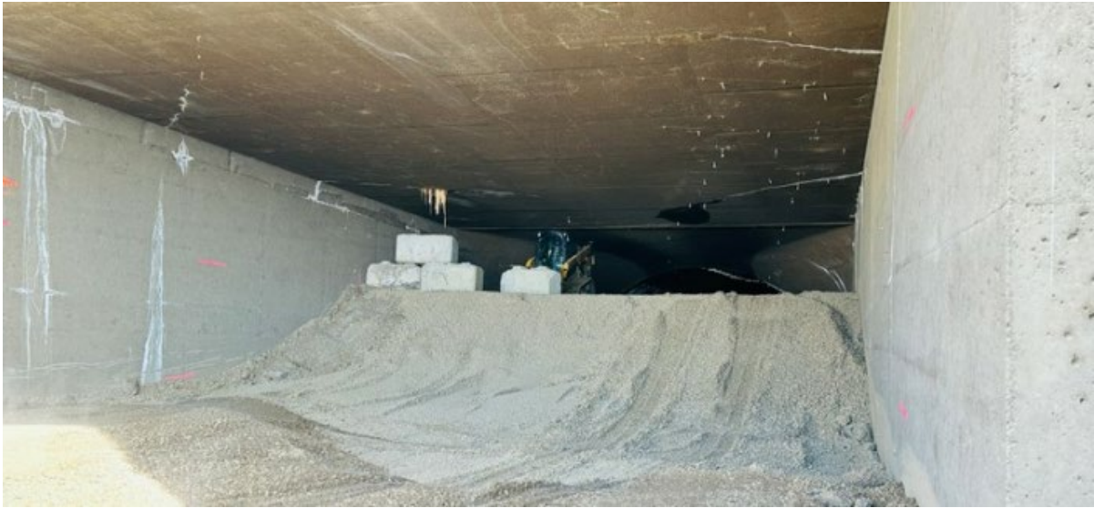
Figure A-28 Diversion Tunnel 1 and 2 Outlet – Setting up Lock Blocks For Backfill (March 2026)
