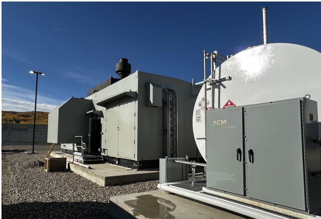
Figure A-25 Spillway Diesel Generator (January 2026)
