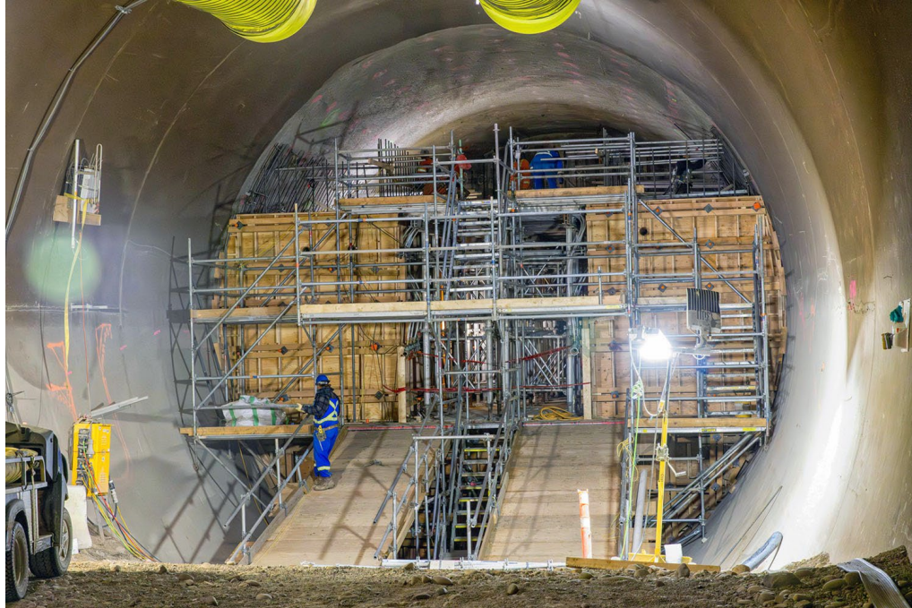
Figure A-10 Construction of the concrete plug for the Diversion Tunnel 1 backfilling (November 2025)
