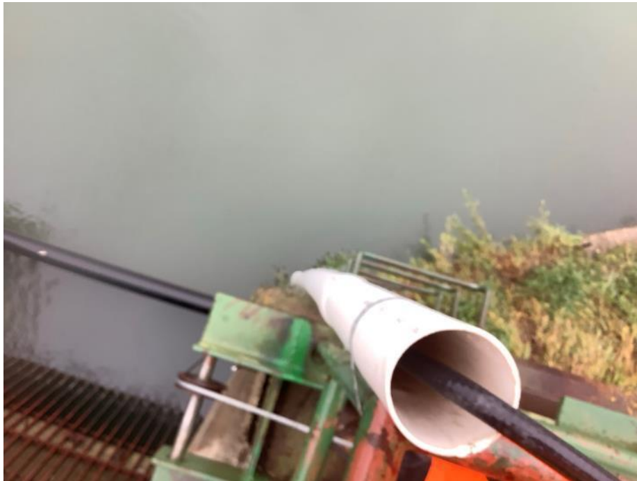
Figure 1. PVC pipe attached to the upstream wingwall of the McMahon Gas Plant intake forebay which contains the Analite turbidity sensor and the TidbiT water temperature sensor.
