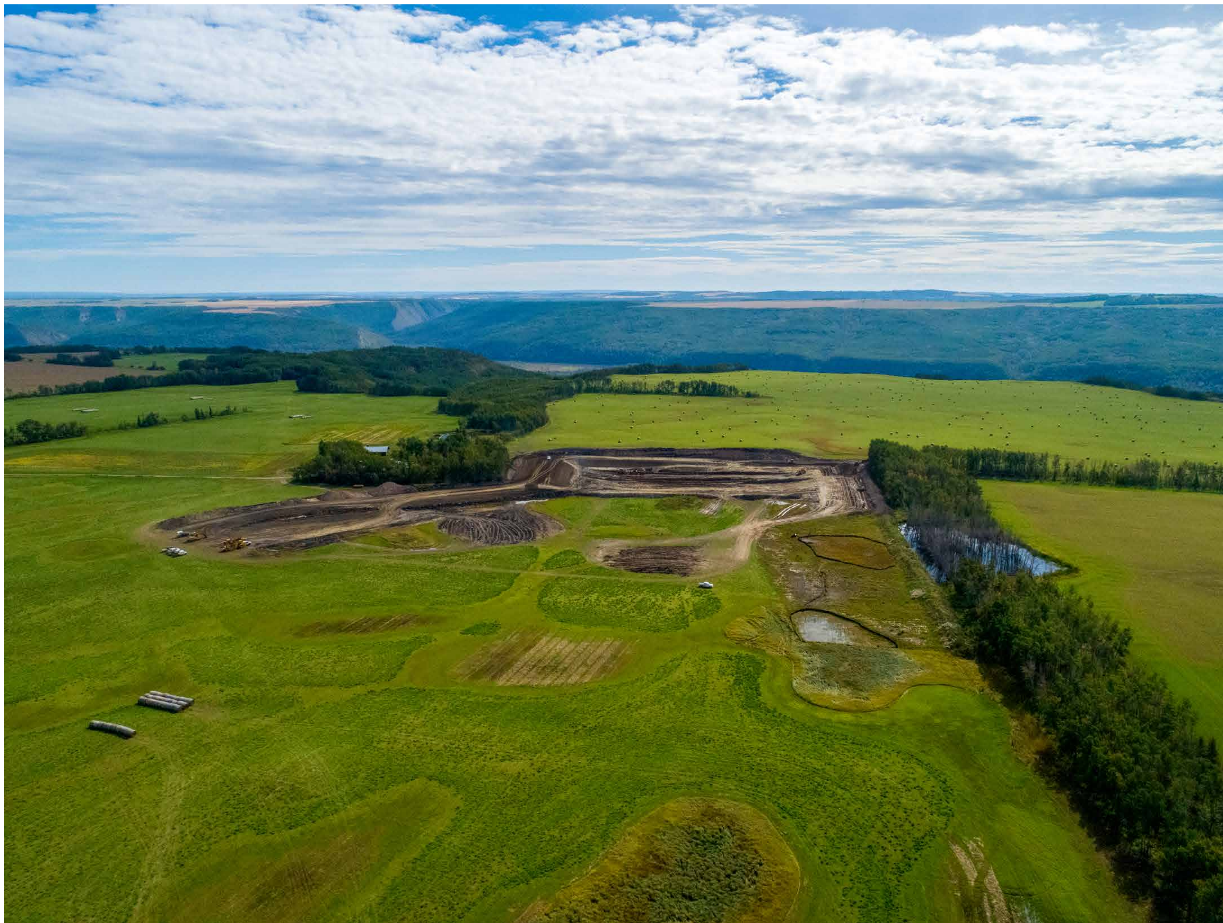
The land is contoured and excavated near Golata Creek to create new wetlands.
