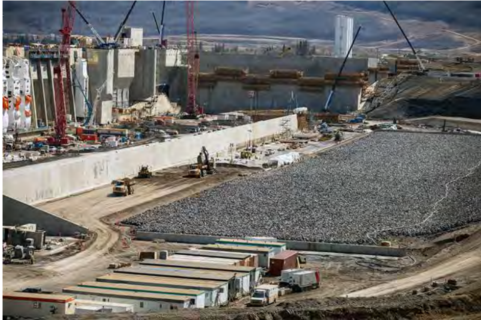
Figure A-1 A partially completed section of the approach channel lining, with riprap cover and granular fill | April 2023
