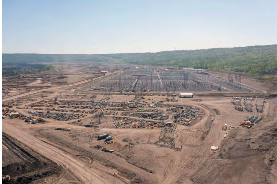
Figure A-4 The 500-kilovolt transmission towers are installed in the substation and ready to be connected to the generating station | May 2023
