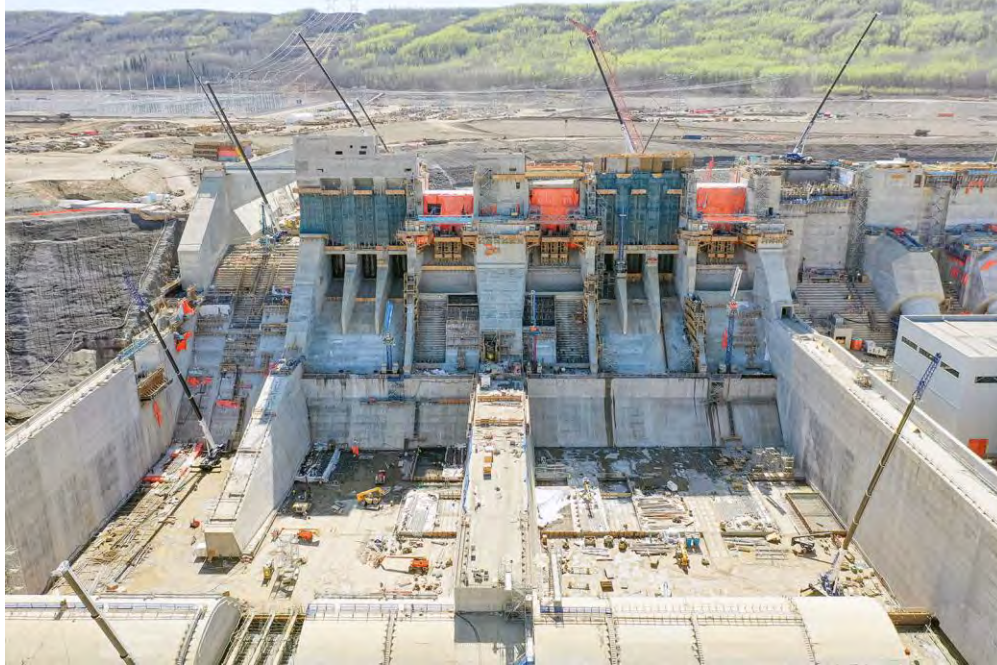
Figure A-6 Two mechanical spillways, operated with gates, will manage flows from the reservoir. The auxiliary spillway is on the left | May 2023
