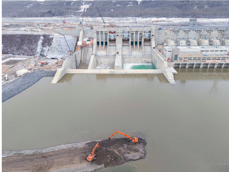
Figure A-3 Spillway construction is completed. Installation of spillway gates continues | November 2023
