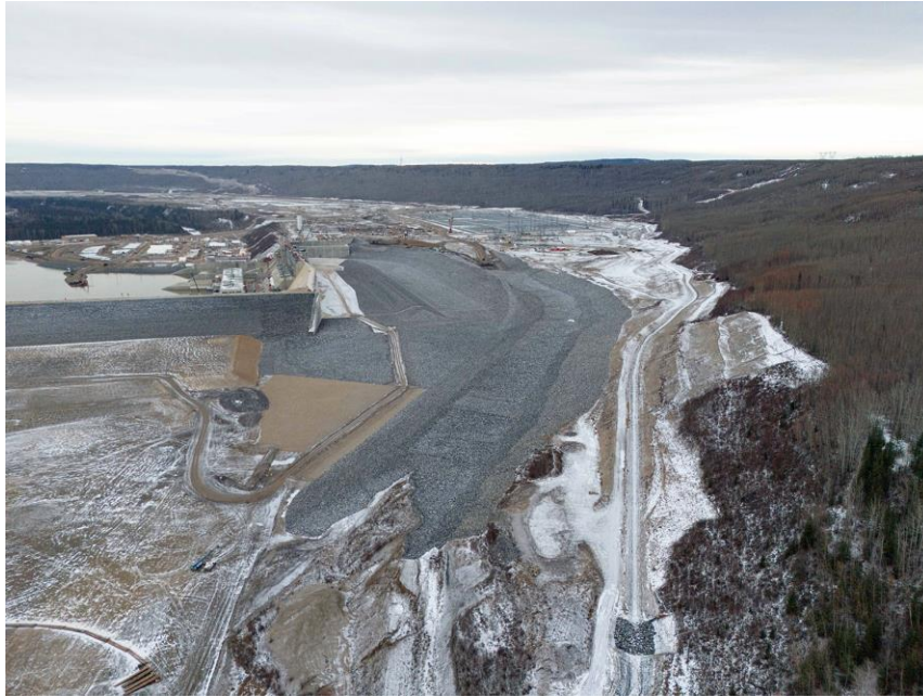
Figure A-5 Riprap placement is substantially completed in the upstream part of the dam, reservoir area, and approach channel | November 2023
