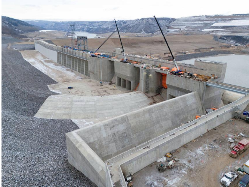
Figure A-7 The approach channel is completed. Water will flow down the channel and enter the intakes, where trash racks have been installed to capture any debris. The auxiliary spillway channel is seen in the foreground | November 2023
