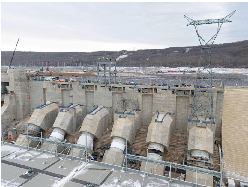
Figure A-4 The first of three transmission towers on top of one of the penstock units | November 2023
