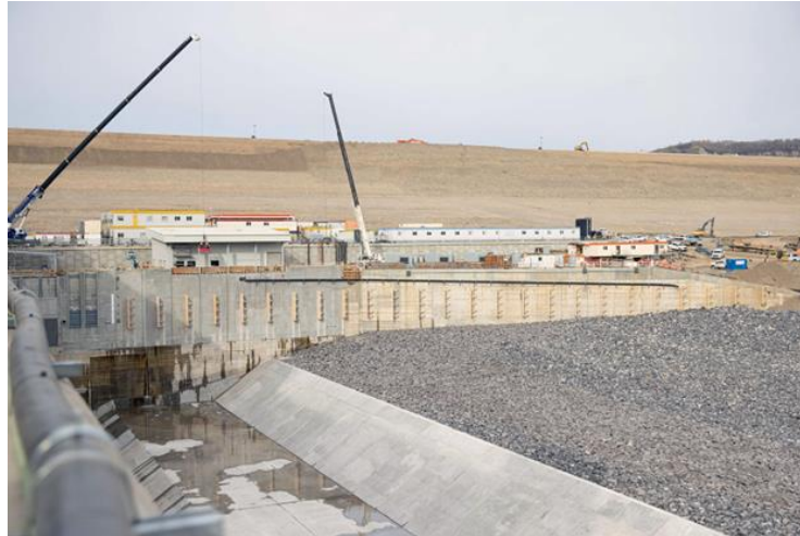
Figure A-1 The permanent upstream fishway facility. In the future, fish travelling upstream to spawn will be attracted to the fast water of the tailrace where they will enter the permanent upstream fishway | October 2023
