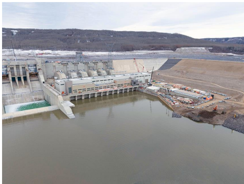
Figure A-6 With the right bank cofferdam removed, the water from the Peace River fills the tailrace area | November 2023
