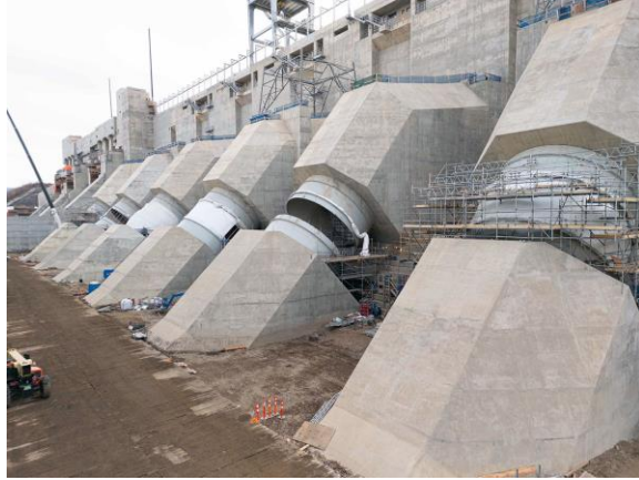
Figure A-9 Concrete placements are complete for the six penstocks. Workers are in the process of installing the flexible couplings, which will join the lower and upper sections of the penstocks together to allow for movement between the lower and upper penstock sections | November 2023
