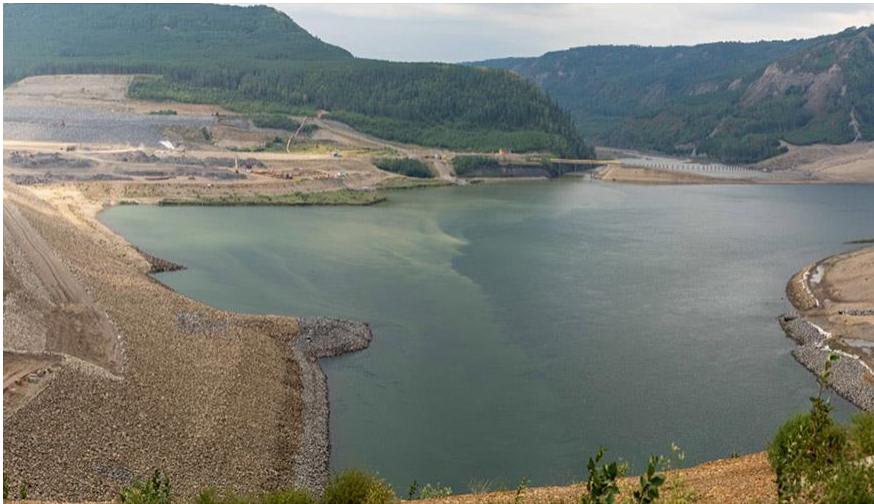
The Site C dam with the reservoir in the background on August 29, 2024. See more photos and video of reservoir fill in our gallery.
