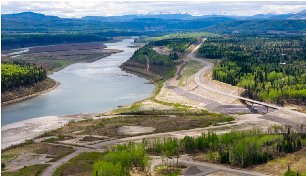
The newly realigned Highway 29 and Lynx Creek Bridge. See more construction photos in our gallery.
