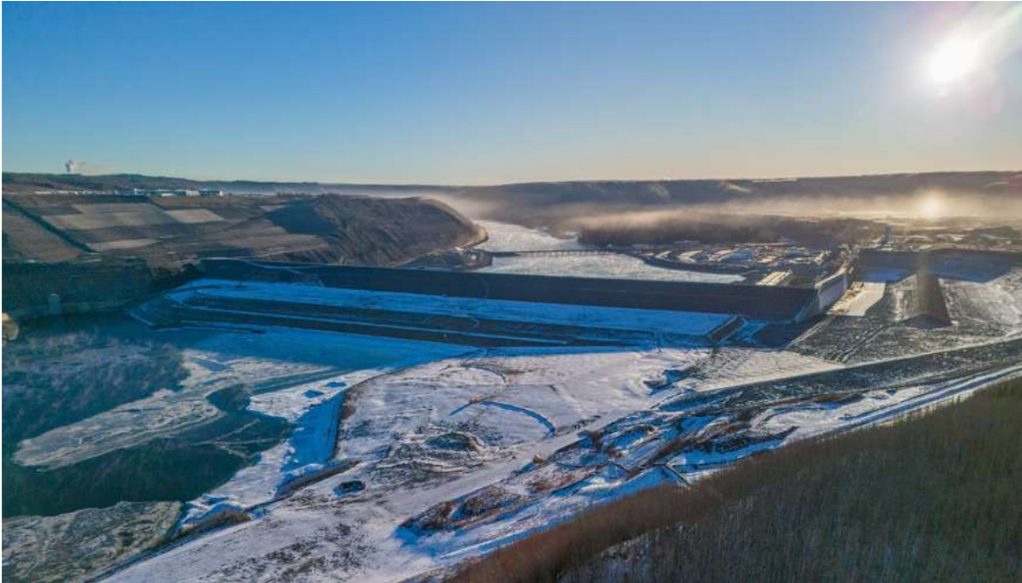
Sunrise at Site C over a snowy powerhouse and earthfill dam. See more construction photos in our gallery.
