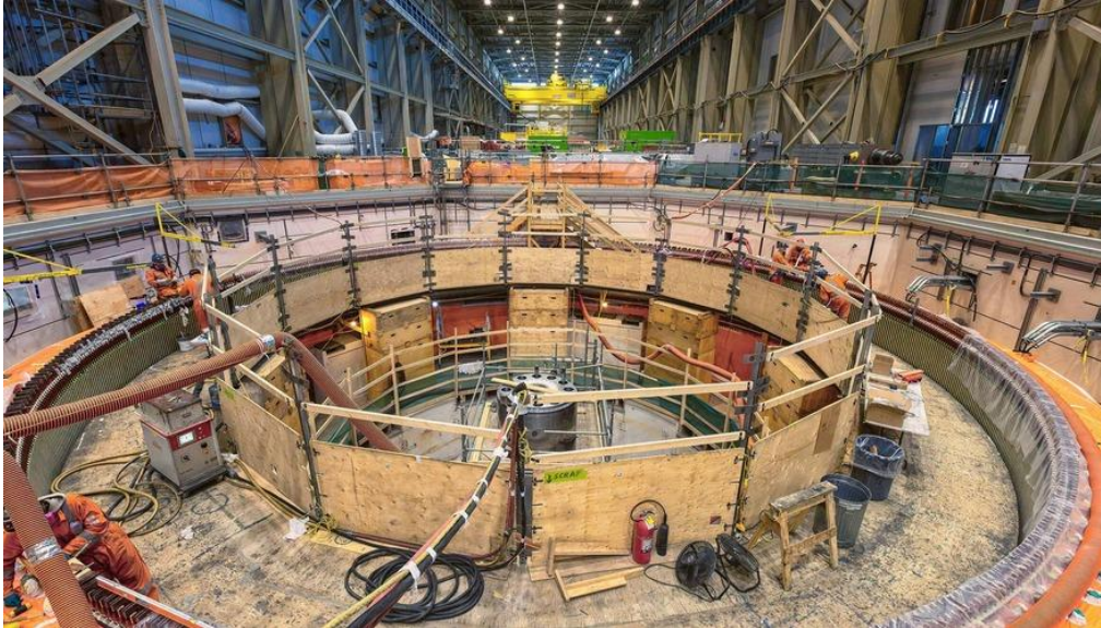
Inside the powerhouse, Unit 6 stator nearing completion. See more construction photos in our gallery.
