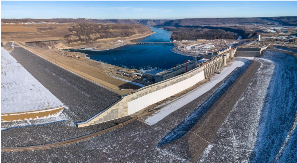
Rip rap placement in the approach channel is complete. See more construction photos in our gallery.
