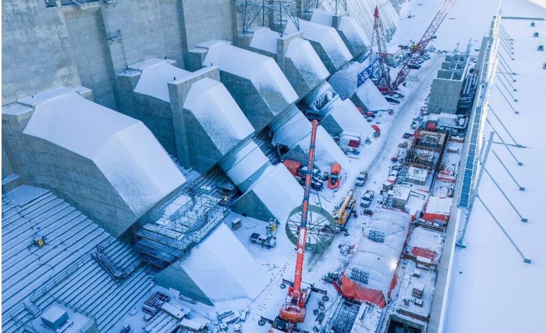
The flexible coupling is suspended on cranes and rotated in the air to a vertical position. See more construction photos in our gallery.
