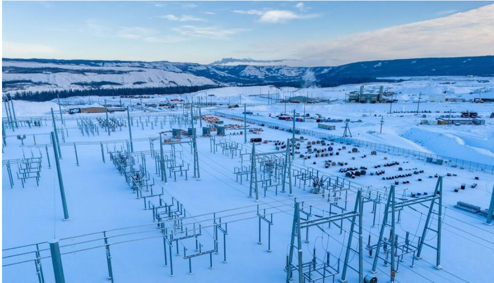
Fresh snow covering the Site C substation. See more construction photos in our gallery.
