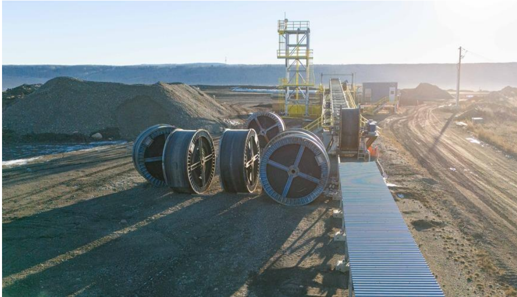
Decommissioning of the five-kilometre-long conveyor belt will continue over the winter through next summer. See more construction photos in our gallery.
