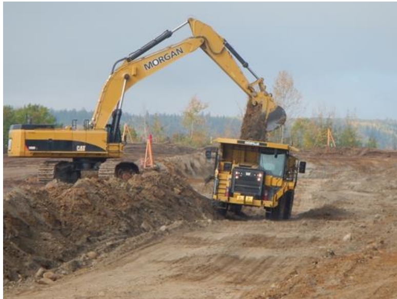
Figure A-2 Excavation of Material; Part of the Left Bank Stabilization on the North Bank of the Site C Dam Site
