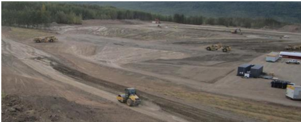
Figure A-5 Work on Access Roads and Site Preparation for the Worker Camp
