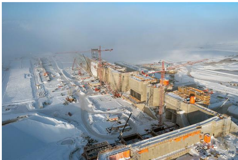
Figure A-2 The upstream wall of the passive spillway (foreground) where water enters the spillway | January 2023
