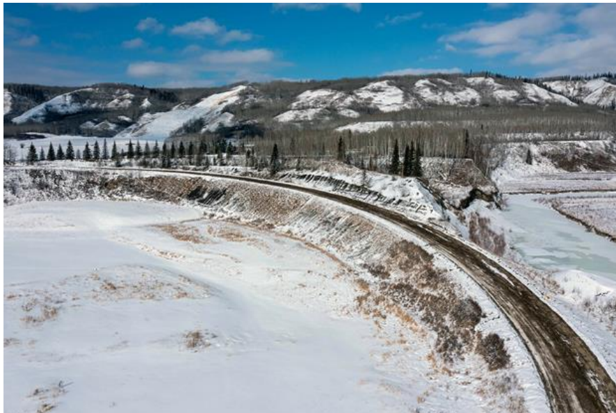
Figure A-10 The asphalt and sub-base gravel from the original Farrell Creek section of Highway 29 has been broken and hauled away to be ground and re-used in future road construction | March 2023
