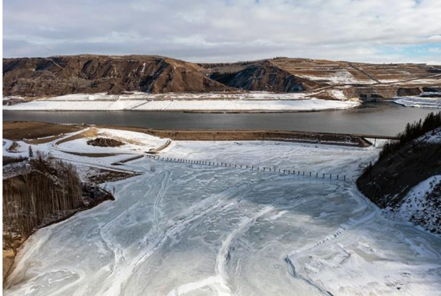
Figure A-9 Where the Moberly and Peace rivers meet upstream of the dam (foreground), the debris boom can be seen, along with the inlet portals for the diversion tunnels (top right) where the river flows around the dam | March 2023
