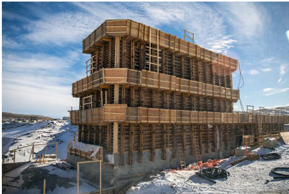
Figure A-8 The end wall of the auxiliary spillway as it transitions into the slurry wall. This is a trench filled with a concrete mix and rebar (slurry) down to bedrock to prevent water seepage | March 2023
