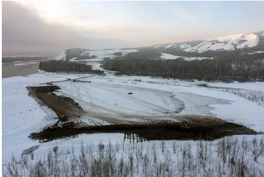
Figure A-1 Phase 1 of the P6 island (an island in the Peace River near Old Fort) reclamation work was completed in mid-January 2023. The island's original soil has been spread over the disturbed areas to allow for growth of seedlings which will be planted in spring 2024 | January 2023
