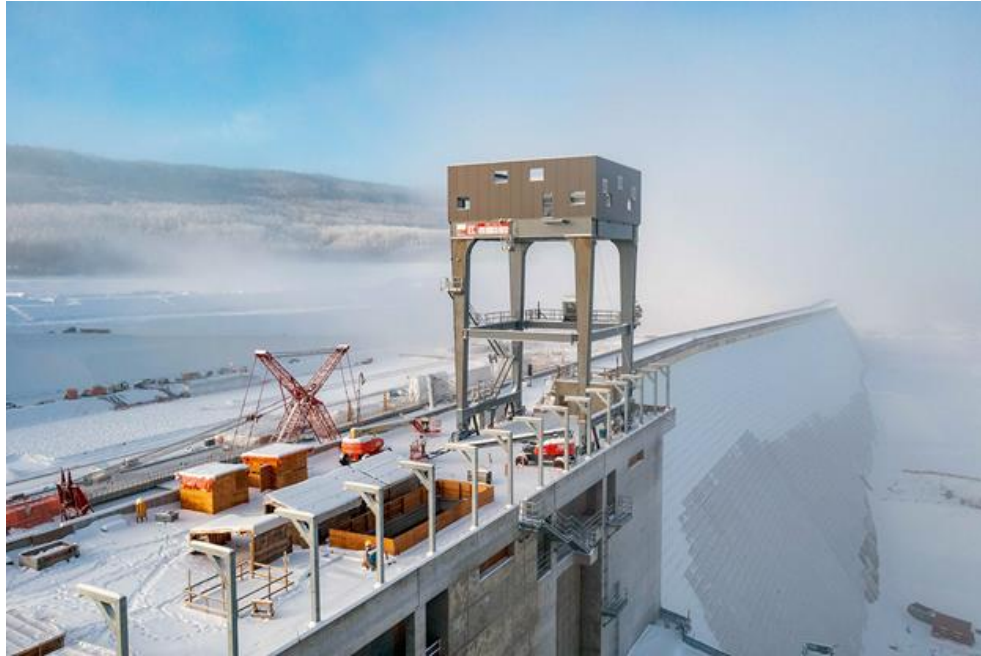
Figure A-3 Assembly of the permanent gantry crane, used for heavy lifts, located above the intakes for the generating units | January 2023
