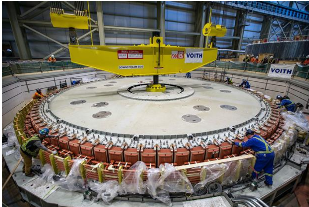
Figure A-6 Unit 1 rotor is lowered into position inside the unit 1 stator | February 2023
