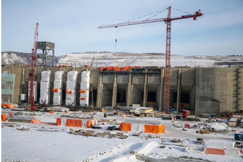
Figure A-7 The unit 2 and 3 trash rack guides are under the winter hoardings and work continues to complete the intakes for units 4 and 5 | March 2023
