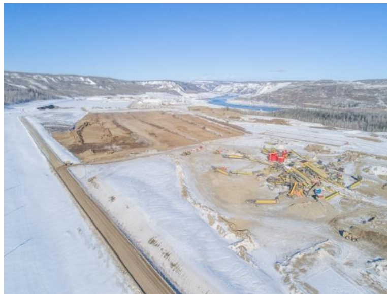
Figure A-4 Aerial View of the South Bank, Facing Northwest with the Crusher Plant in the Foreground. Photo taken February 28, 2018.
