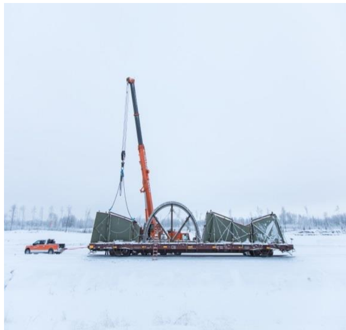
Figure A-2 The Turbines and Generators Contractor Delivering Equipment to their Work Area. Photo taken January 24, 2018.
