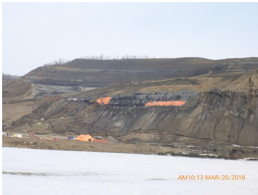
Figure A-8 Overview of Left Bank Excavations and Inlet Portal Works. Photo taken March 20, 2018.
