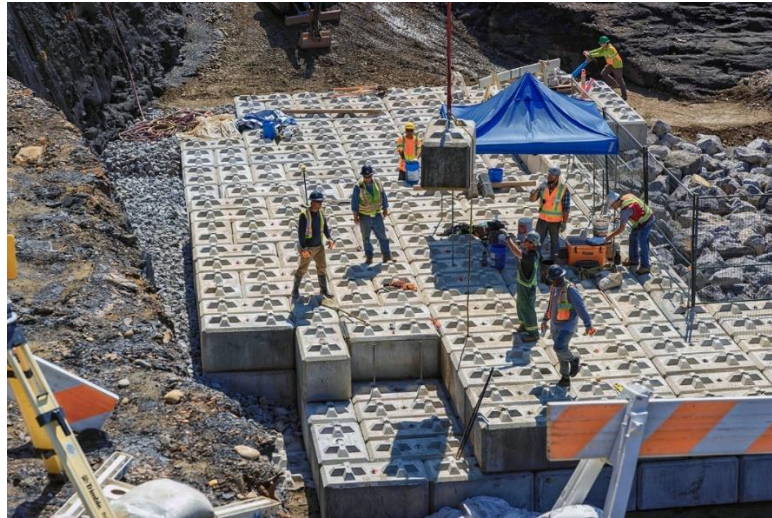
Figure A-1 The placement of concrete lock-blocks to construct the left bank drainage wall. Each concrete block weighs 2,000 kg | July 2024
