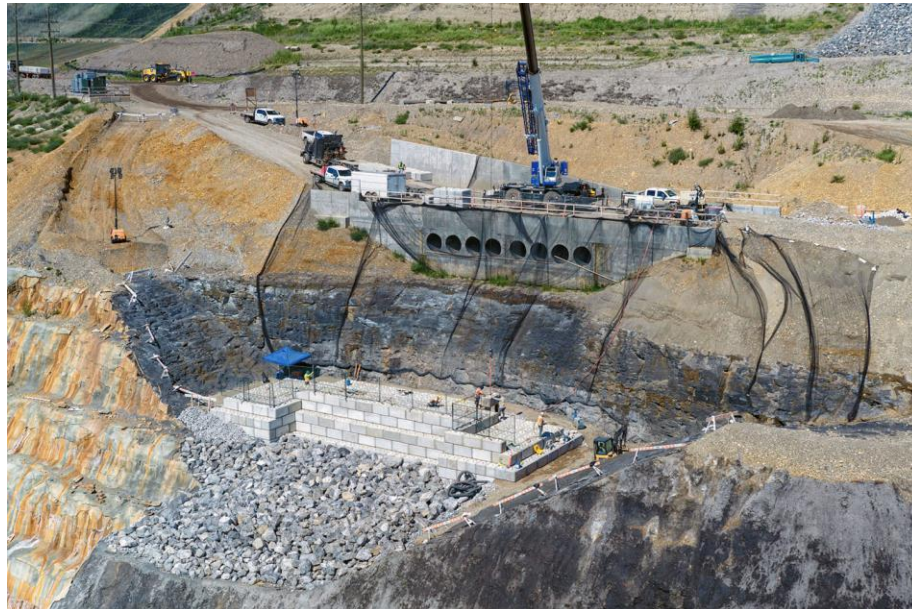
Figure A-4 The left bank drainage structure includes a rip rap lined channel that directs the flow of water through the box culvert. Fifteen layers of lock-blocks will complete the drainage structure to direct water into the reservoir and away from the dam | July 2024
