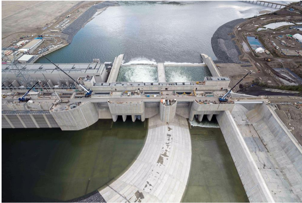
Figure A-8 Water flows through the Site C spillways during the reservoir filling process | September 3, 2024
