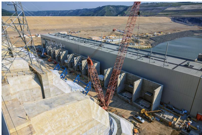
Figure A-2 The main step-up transformer bays are in groups of three with one spare unit. The bay houses the three step-up transformers that are connected to generating units 1 and 2, and these transformers are connected to the transmission grid. The second set of three step-up transformers are installed and being commissioned | July 2024
