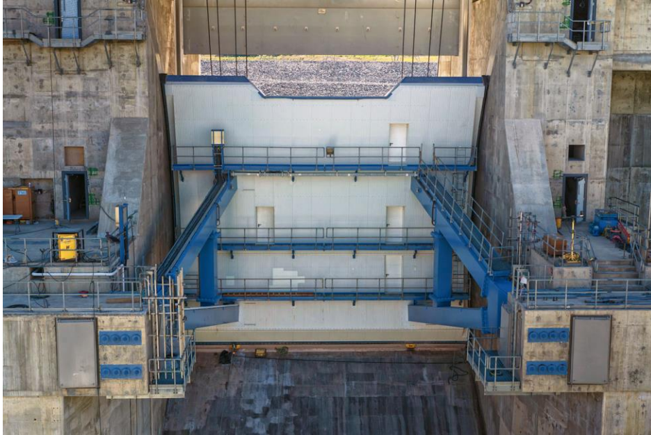
Figure A-5 Concrete finishing work being completed on the door sill of the second spillway operating gate. The spillway gates are lifted by hoist cables and pivot on axis points | July 2024
