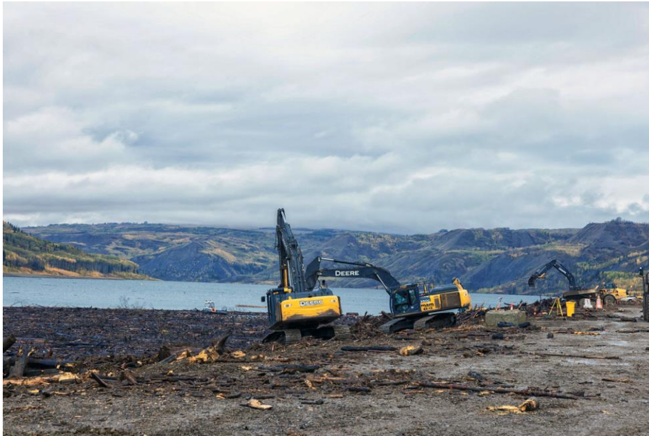
Figure A-9 The removal of wood debris during reservoir filling. This wood debris was collected to a debris removal location near the dam site, and then removed from the reservoir and stockpiled for future use | September 2024
