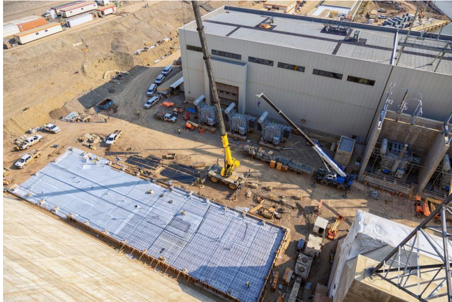
Figure A-3 Formwork and reinforcing steel are in place on the concrete slab to construct the emergency response (ERT) team building | July 2024
